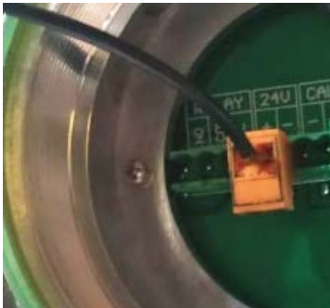
Power DC 24V (orange Terminal)
